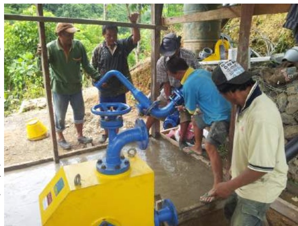
Micro-hydro project in Sabah, Malaysia (Tonibung)
